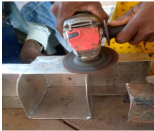
Figure 48. Grinding of the central component
